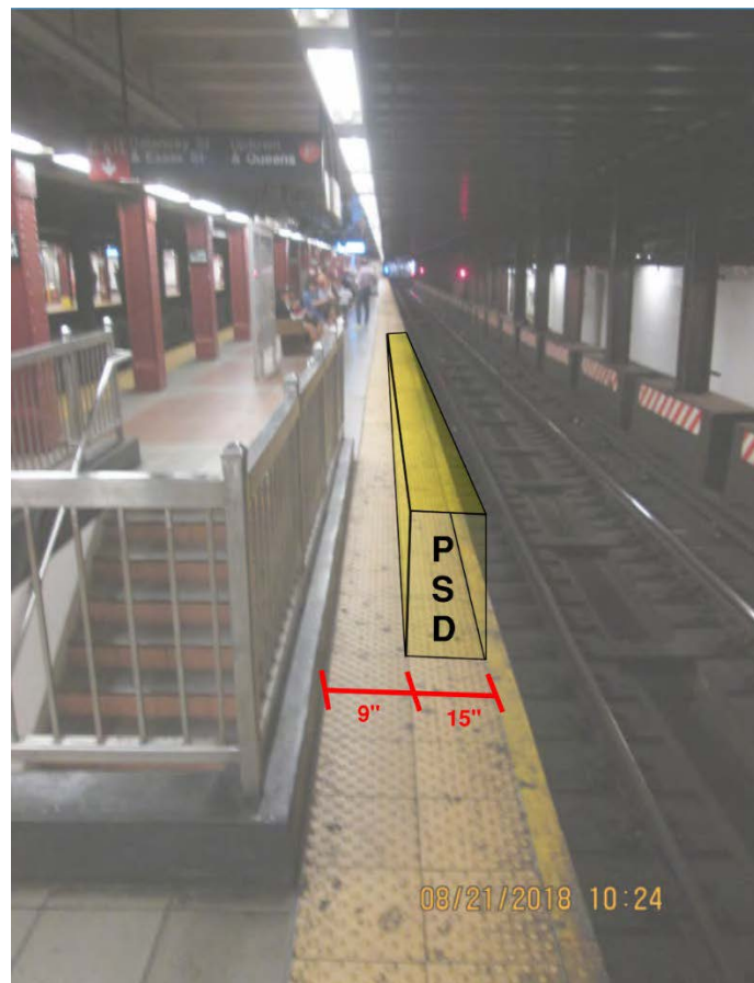
Figure 1 – Non-Compliant ADA condition Essex / Delancey Station
