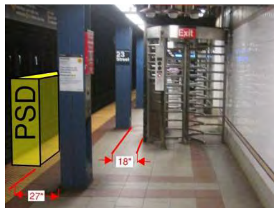
Figure 2 – Non-Compliant ADA condition 23 rd Street
