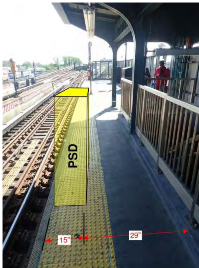
Figure 1 – Non-Compliant ADA condition Rockaway Boulevard
