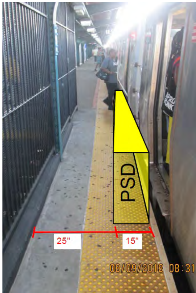
Figure 1 – Non-Compliant ADA condition Kosciusko Street
