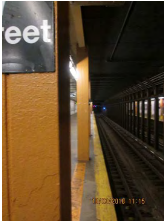
Figure 1 – Columns 1'-2" from the edge 77 th Street Station
