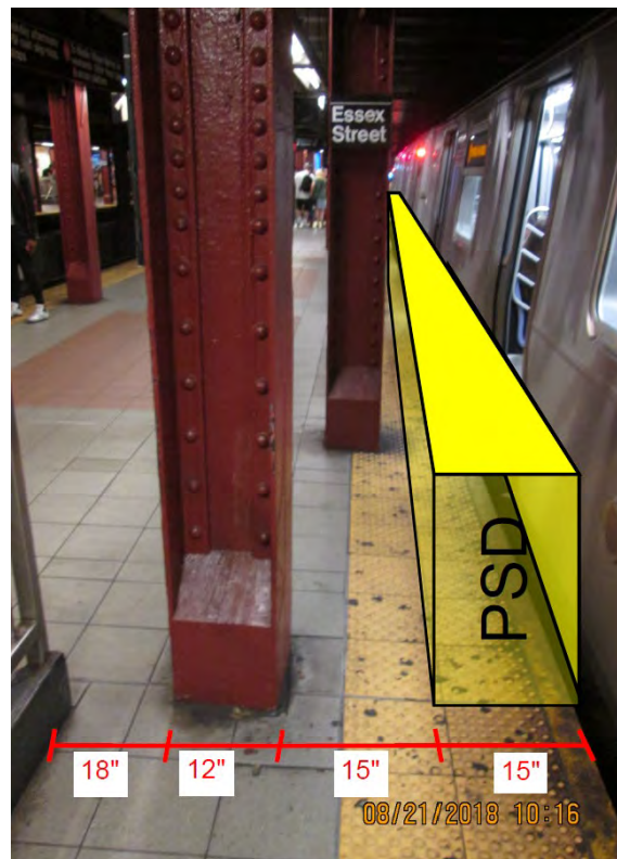
Figure 1 – Non-Compliant ADA condition Delancey Street - Essex Street Station
