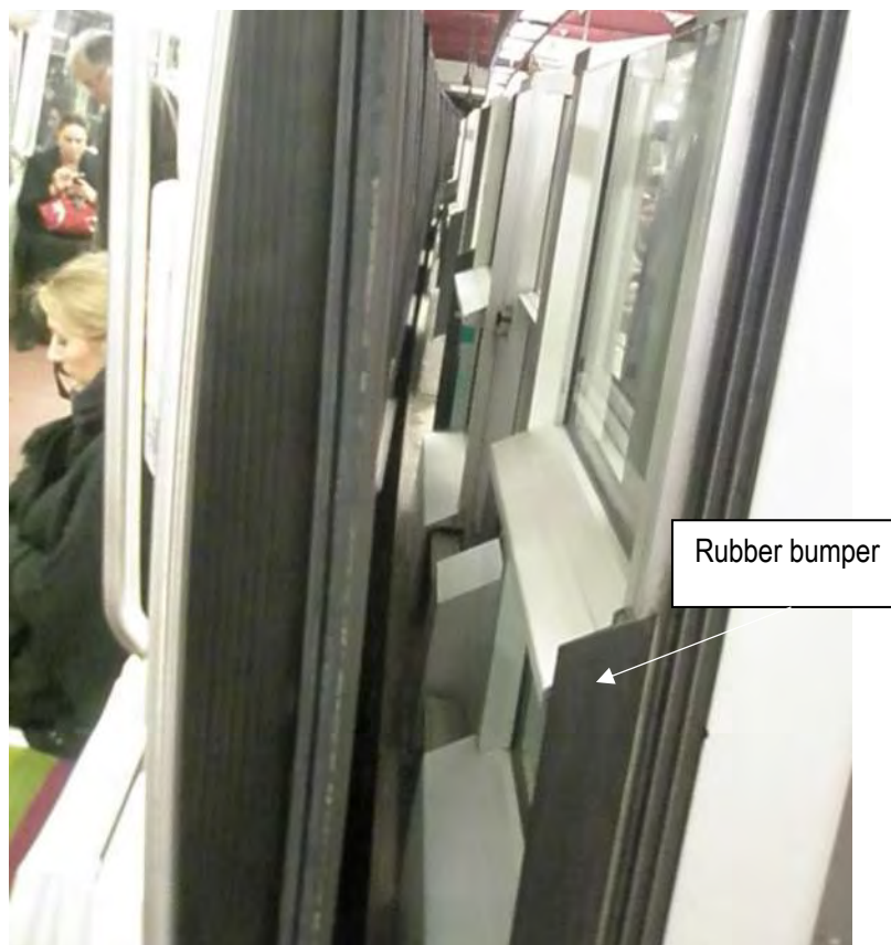
Figure 10 - Rubber bumper on leading edge of platform APG door at bottom of photo
