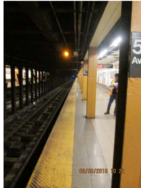
Figure 3 – Signal above platform edge Fifth Avenue Station
