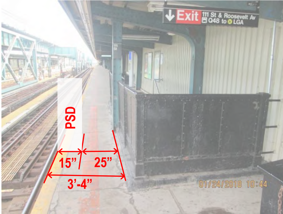
Figure 2 – Typical stair location and platform condition – 111 th Street Station
