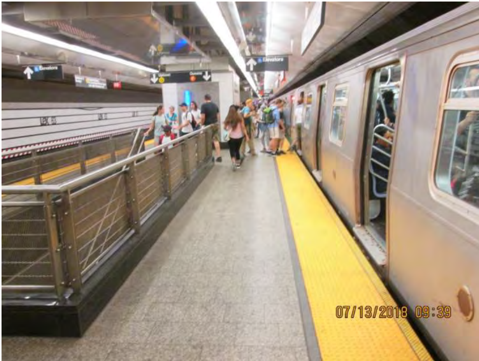
Figure 3 – Platform edge condition on the upper level (Coney Island-bound)- Lexington Ave.-63rd St. Station
