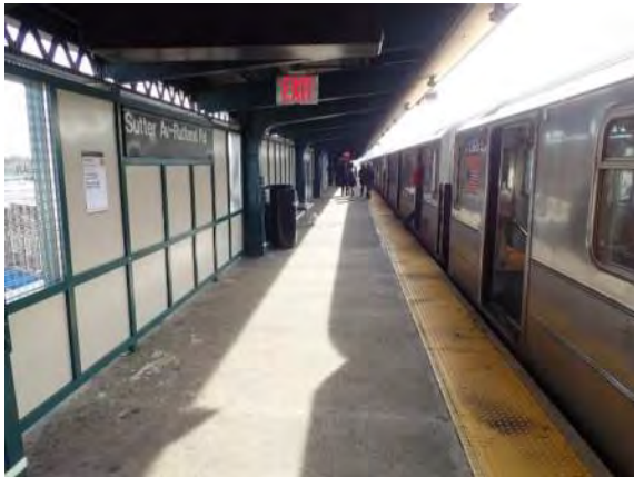
Figure 1 – General Station Condition Sutter Avenue Station
