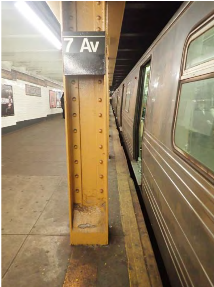
Figure 1 – Column 12” from the edge 7th Avenue Flatbush Avenue Station
