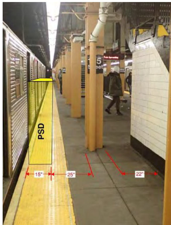
Figure 1 – Non-Compliant ADA condition 145 th Street
