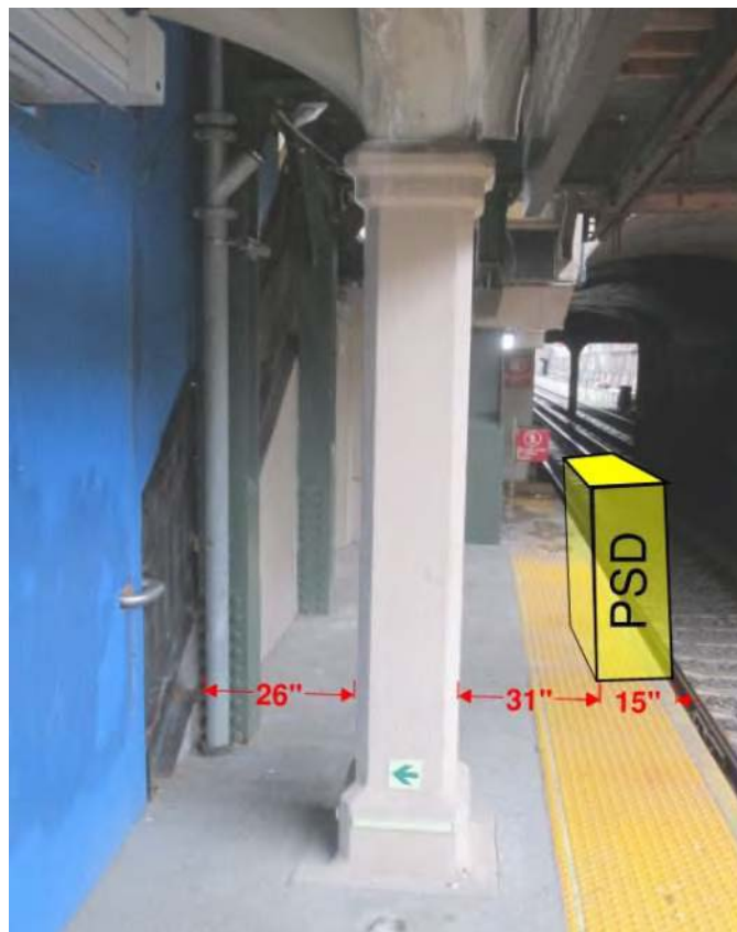
Figure 1 – Non-Compliant ADA condition 18 th Avenue Station
