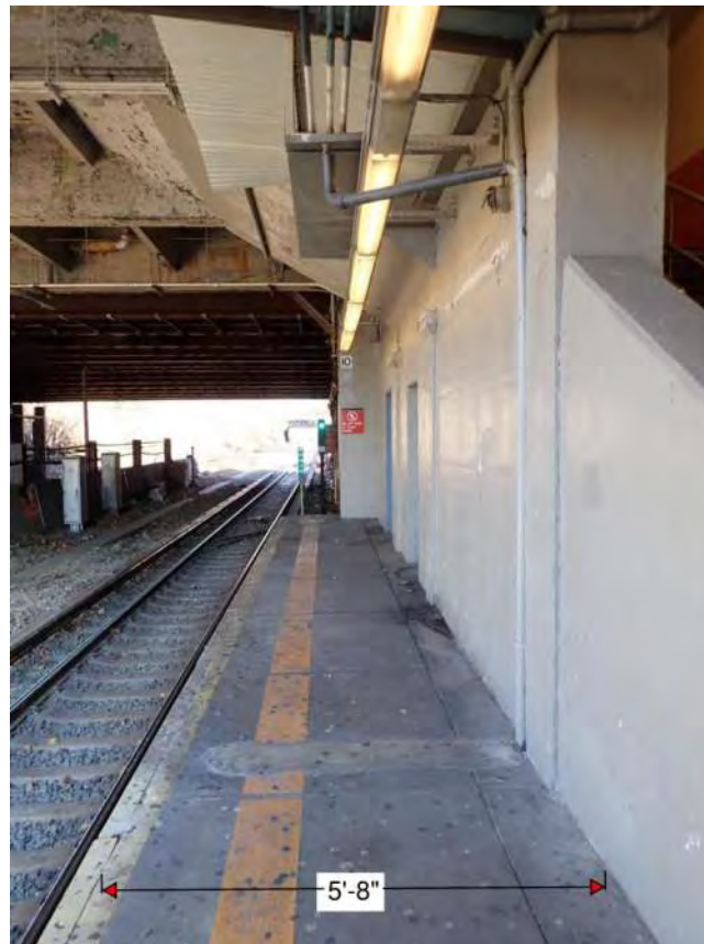
Figure 1 – Area of Non-compliant egress width Gun Hill Road Station
