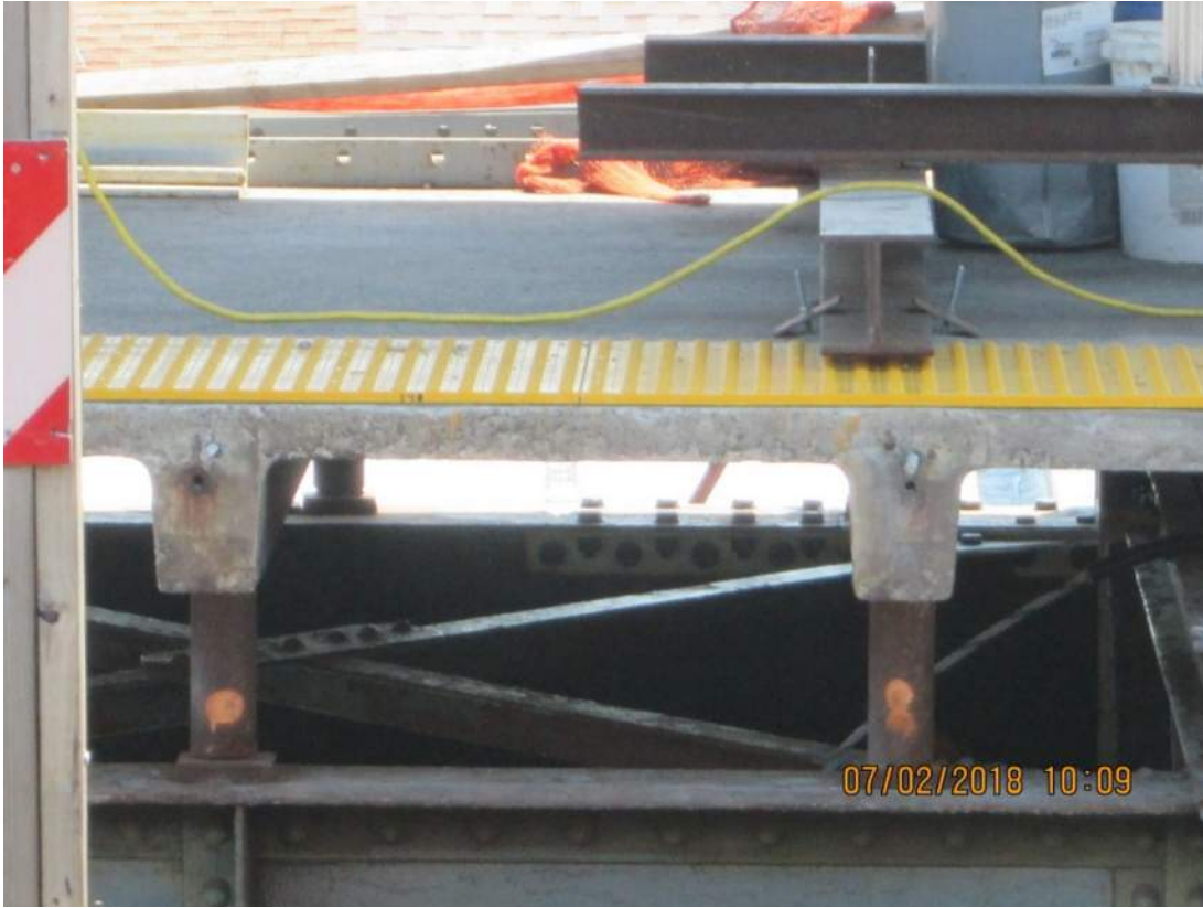
Figure 2– Precast T-Beam platform – Avenue U Station
