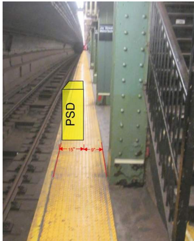
Figure 1 – Non-Compliant ADA condition Jay Street Station
