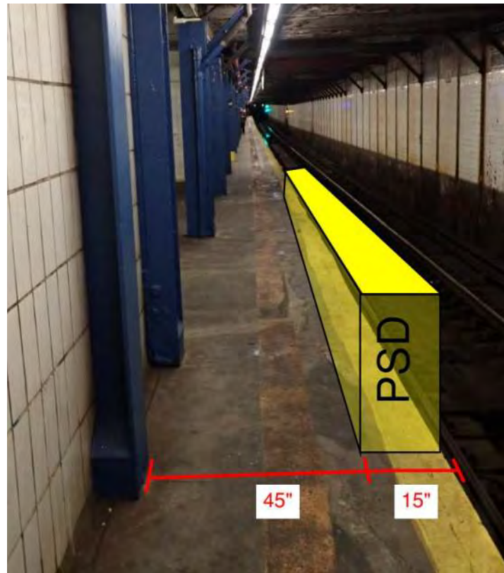
Figure 1 – Non-Compliant code condition 14 th Street Station
