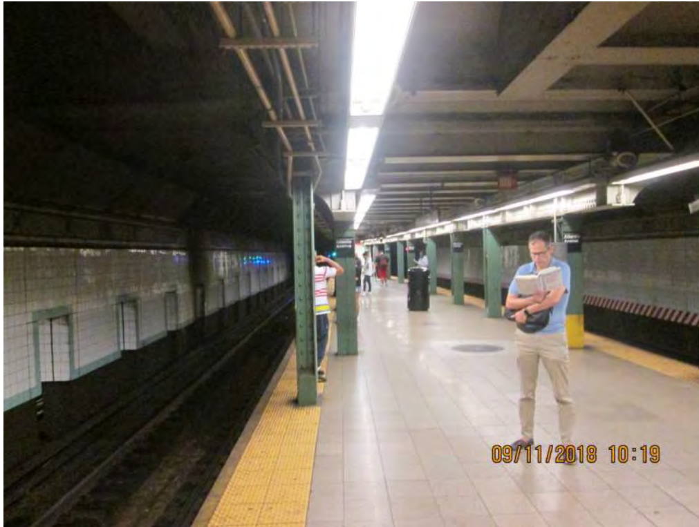
Figure 3 – View of column at platform edge requiring removal and replacement Atlantic Ave Station
