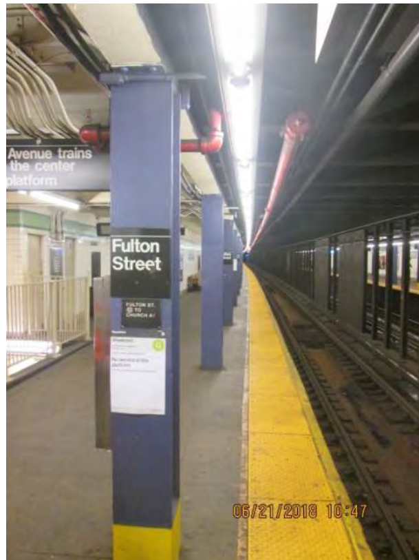
Figure 3 – Typical platform view with standpipe MRN 292: Fulton Street Lafayette Avenue
