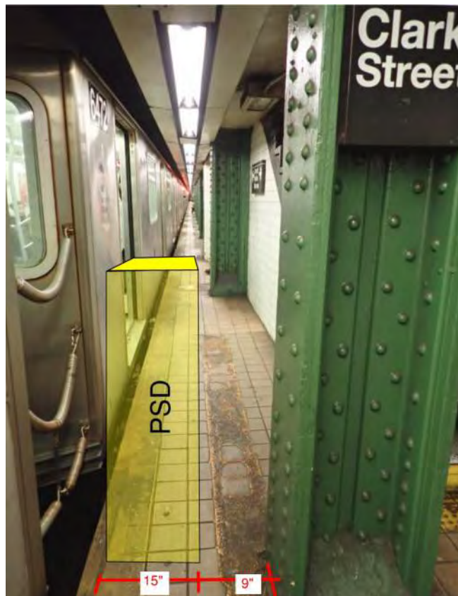
Figure 1 – Non-compliant ADA condition Clark Street Station
