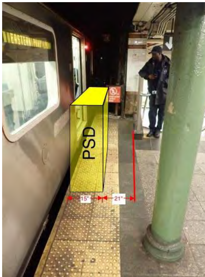
Figure 1 – Non-compliant ADA condition Atlantic Ave Station
