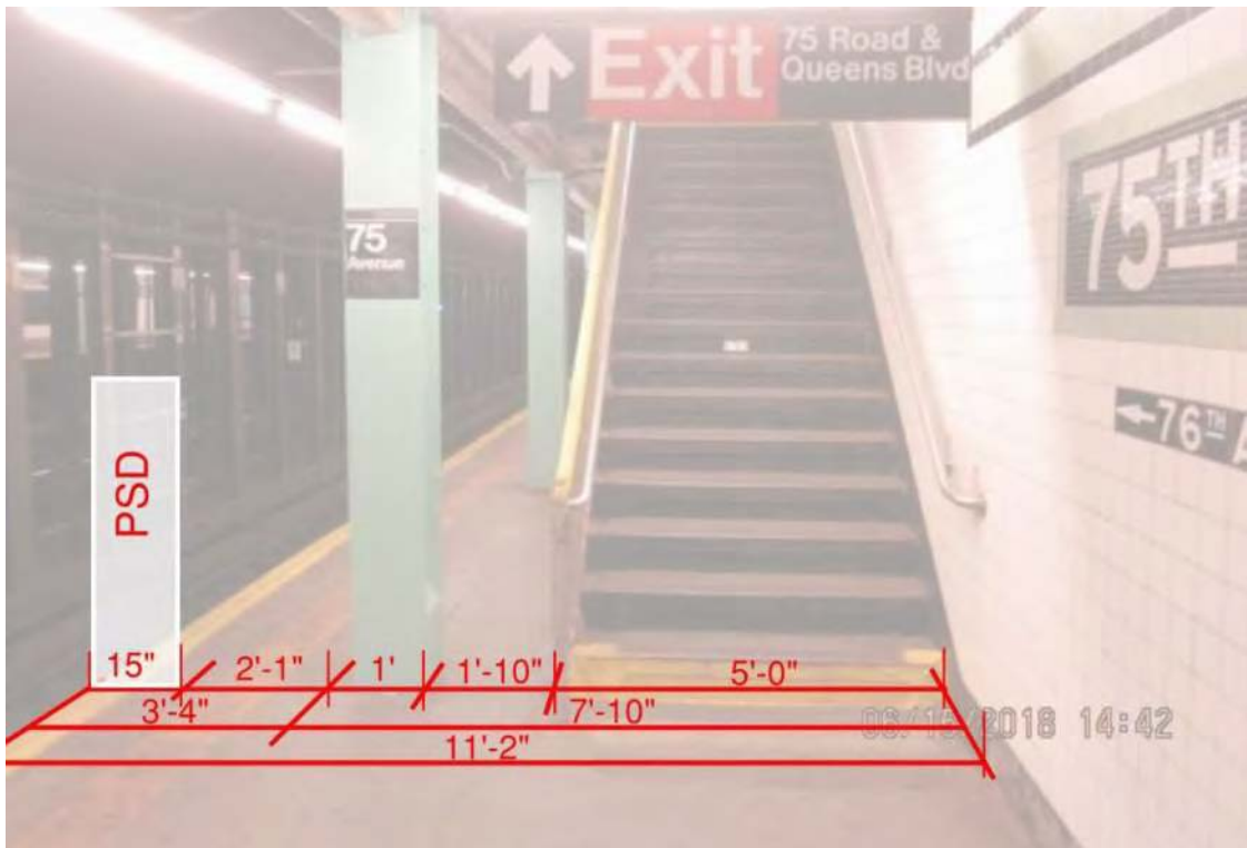
Figure 1 – Non-compliant condition at stairs (typical) - 75 th Avenue
