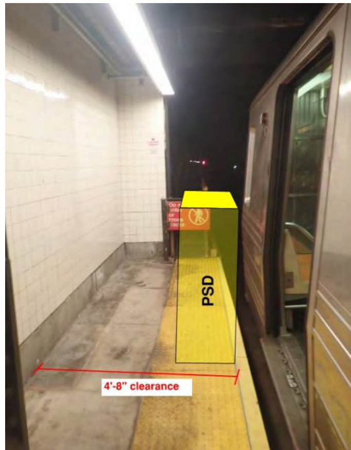
Figure 1 – Non-Compliant ADA condition 72 nd Street Station
