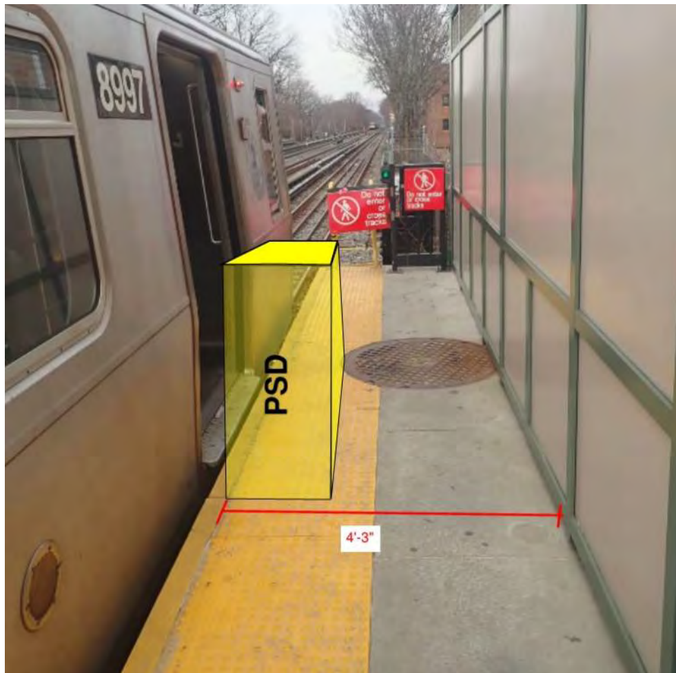
Figure 1 – Non-Compliant egress condition Avenue M Station
