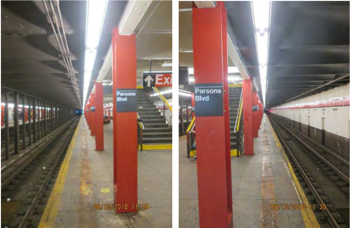
Figure 2 – Typical edge conditions | Express condition (left) and local condition (right)– Parsons Blvd. Station
