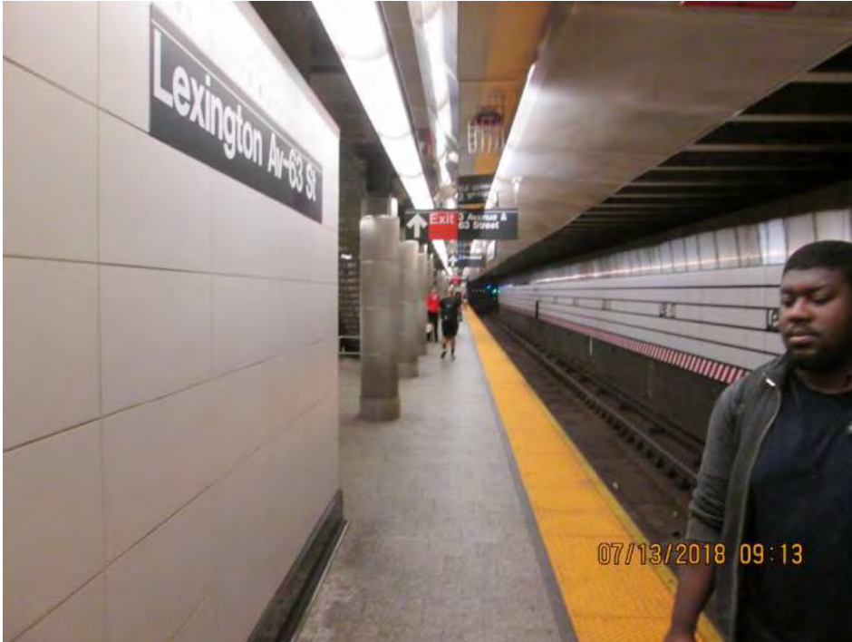
Figure 4 –Platform edge condition on the lower level (96 th Street-bound)- Lexington Ave.-63rd St. Station
