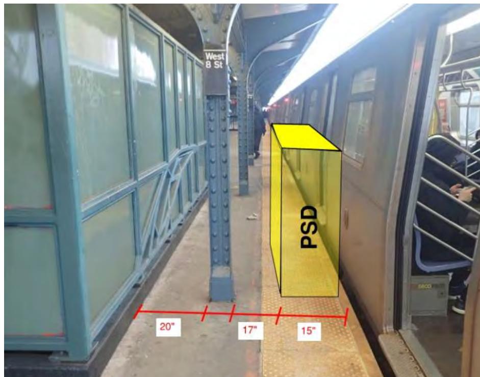
Figure 1 – Non-compliant ADA condition on the Manhattan-bound platform- West 8 th St-NY Aquarium
