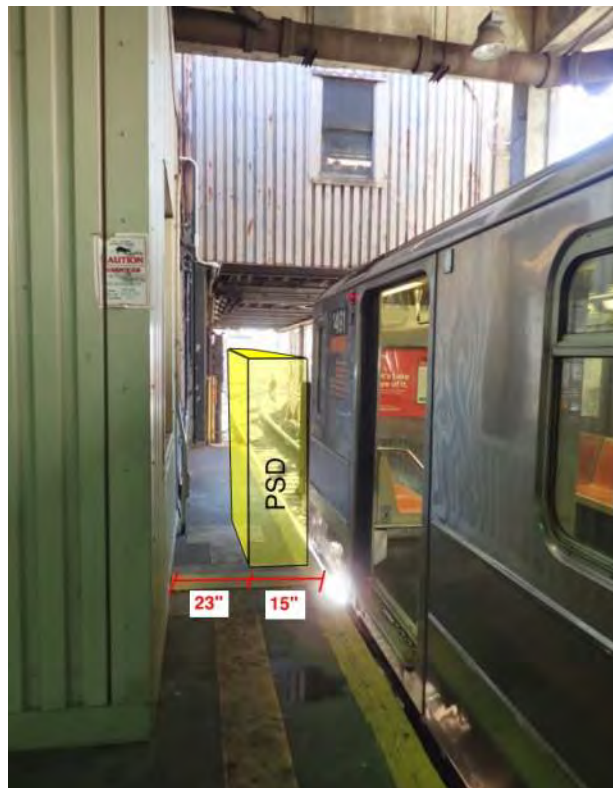
Figure 1 – Non-compliant ADA condition 148 th Street Station
