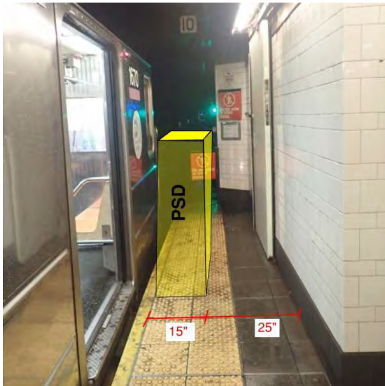
Figure 1 – Non-compliant ADA condition 77th Street Station
