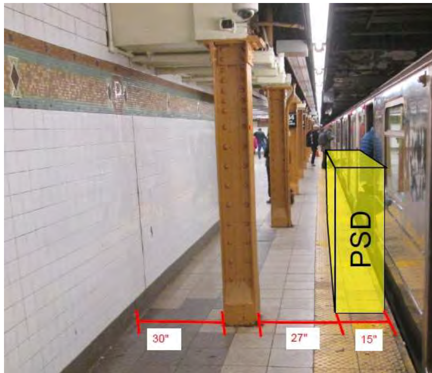
Figure 1 – Non-Compliant ADA condition 34th Street Station
