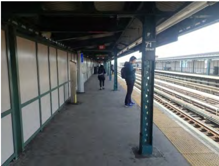
Figure 1 – General Station Condition 71 st Street Station
