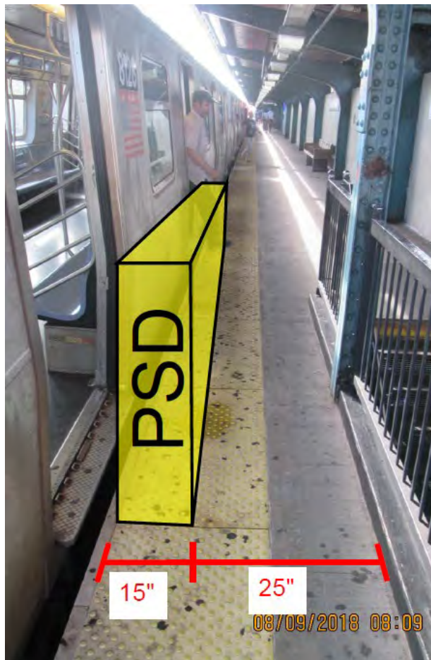
Figure 1 – Non-Compliant ADA condition Gates Avenue
