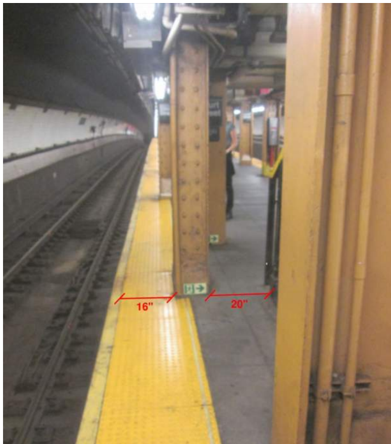
Figure 1 – Obstruction at platform edge Court Street Station
