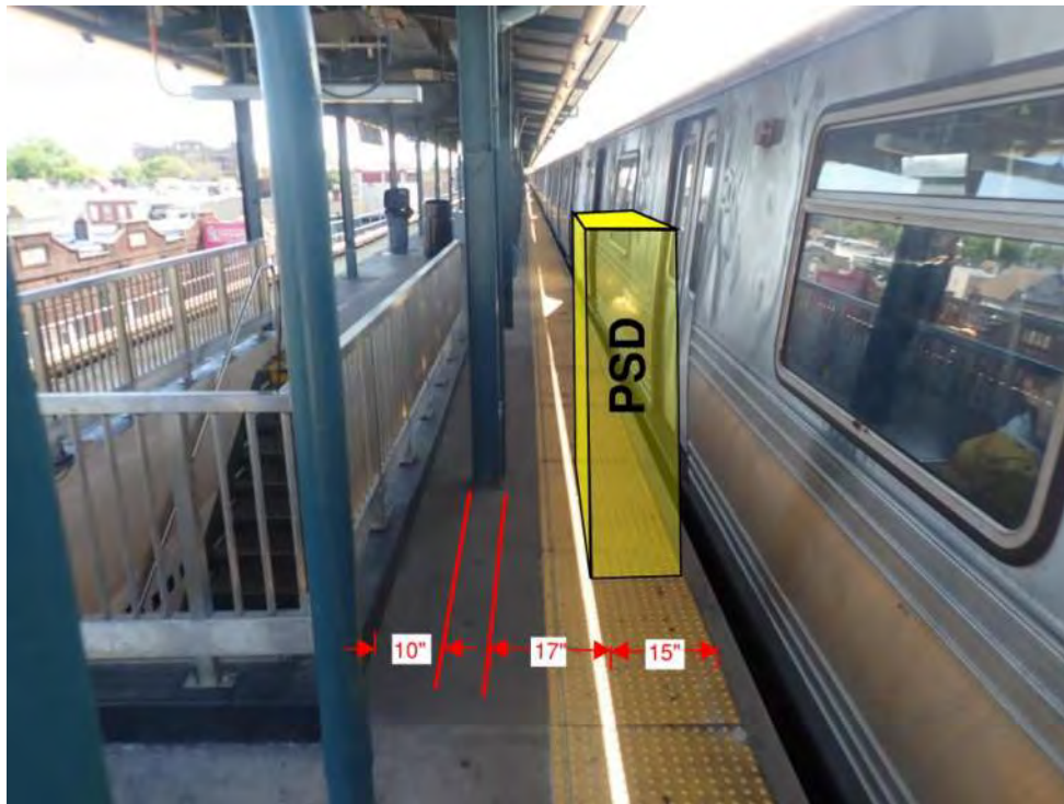
Figure 1 – Non-Compliant ADA condition Lefferts Boulevard
