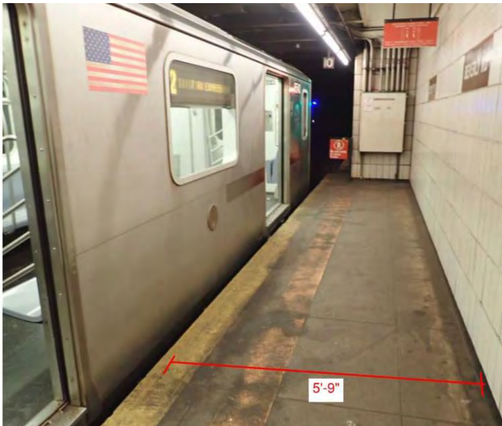
Figure 1 – Non-Compliant egress condition Beverly Road Station
