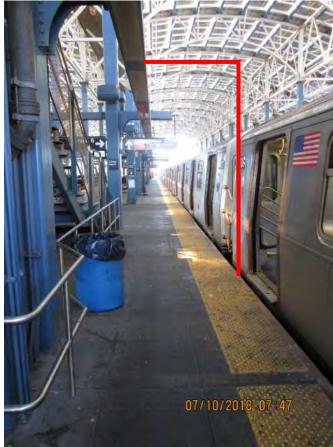
Figure 3 – Typical platform edge condition with line of potential supplementary framing- Coney Island-Stillwell Avenue Station
