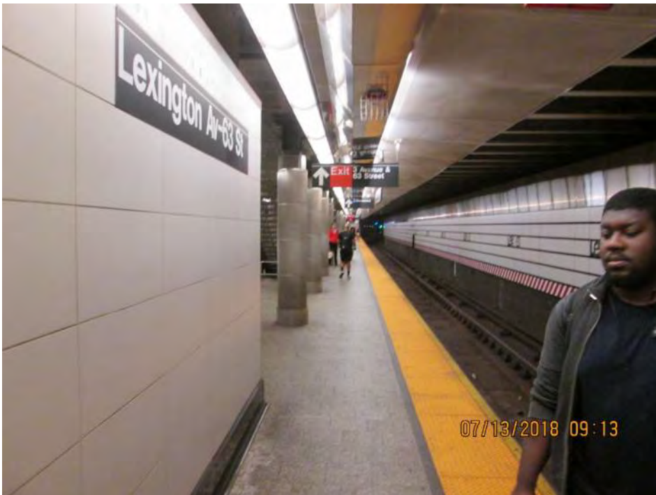
Figure 4 –Platform edge condition on the lower level (Jamaica-bound)- Lexington Ave.-63rd St. Station
