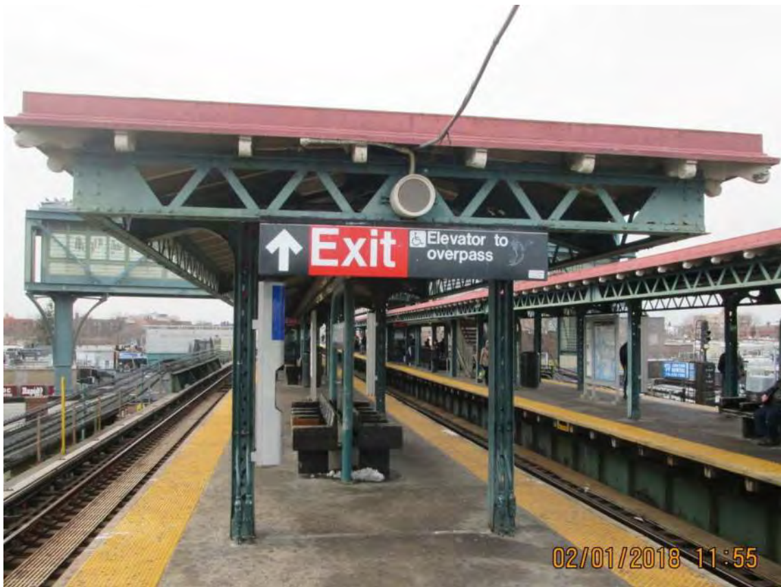
Figure 1– Typical platform condition – Junction Boulevard Station
