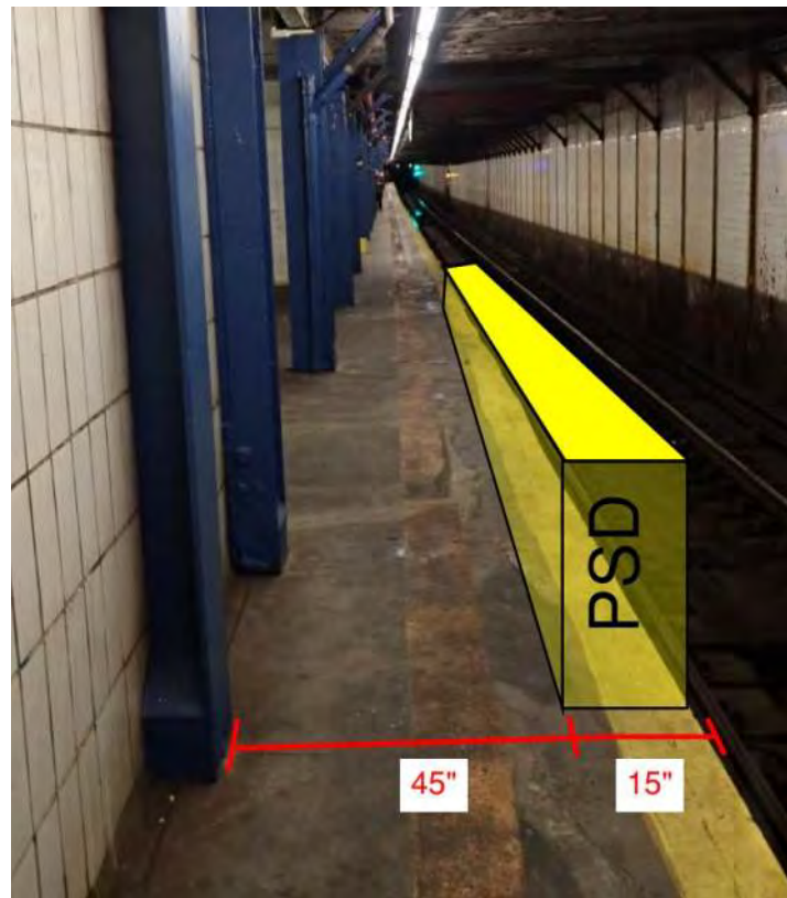
Figure 1 – Non-Compliant egress condition 14 th Street Station
