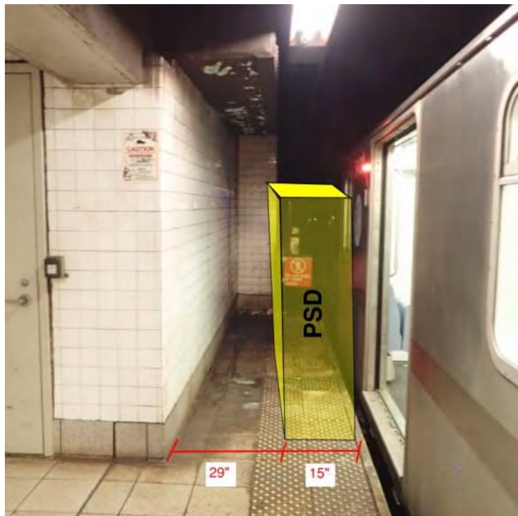
Figure 1 – Non-compliant ADA condition Grand Army Plaza Station
