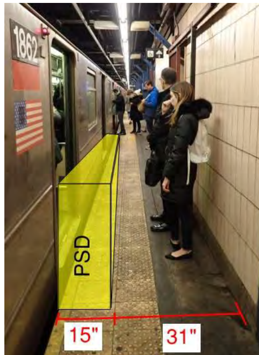
Figure 1 – Non-compliant ADA condition Chambers Street Station
