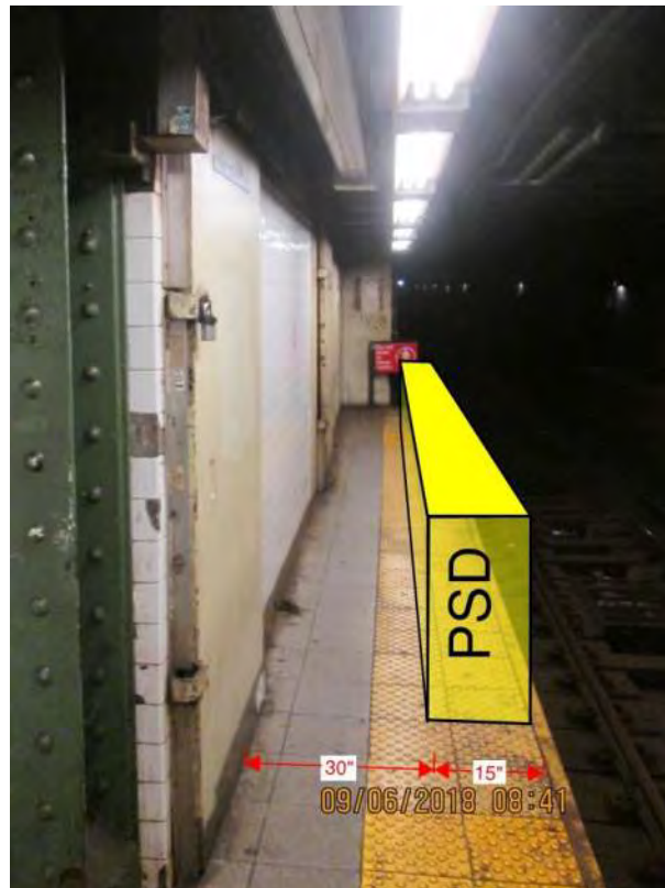
Figure 1 – Non-Compliant ADA condition Lexington 59 th Street Station
