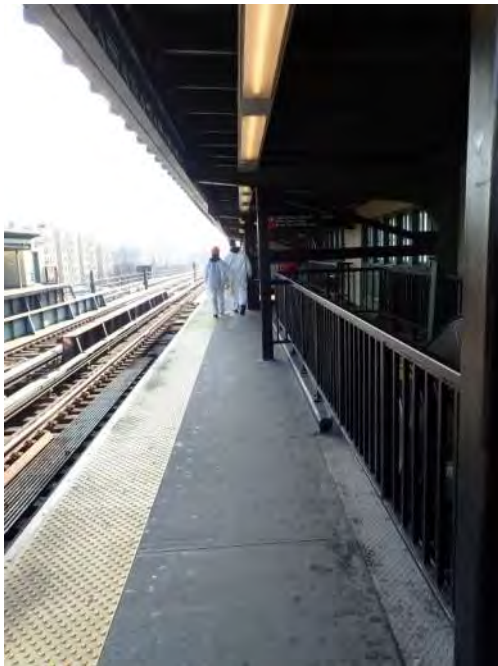
Figure 1 – General Station Condition Pelham Parkway Station
