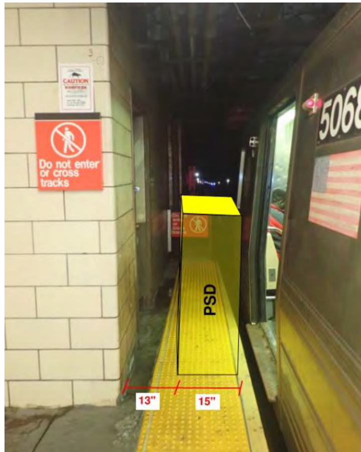
Figure 1 – Non-Compliant ADA condition 103 rd Street
