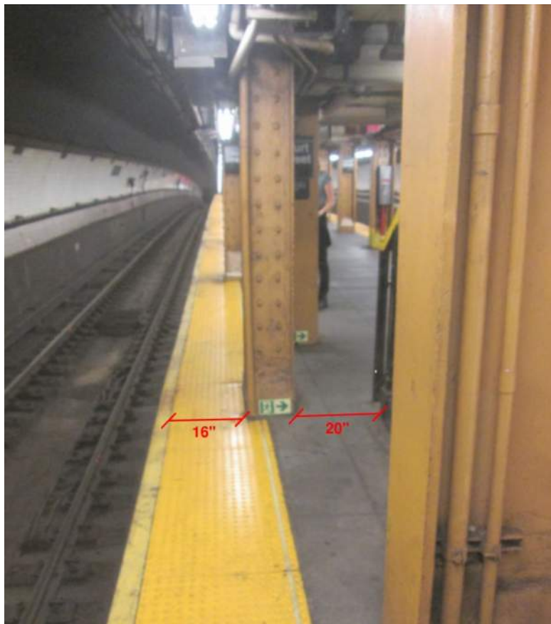
Figure 1 – Obstruction at platform edge Court Street Station
