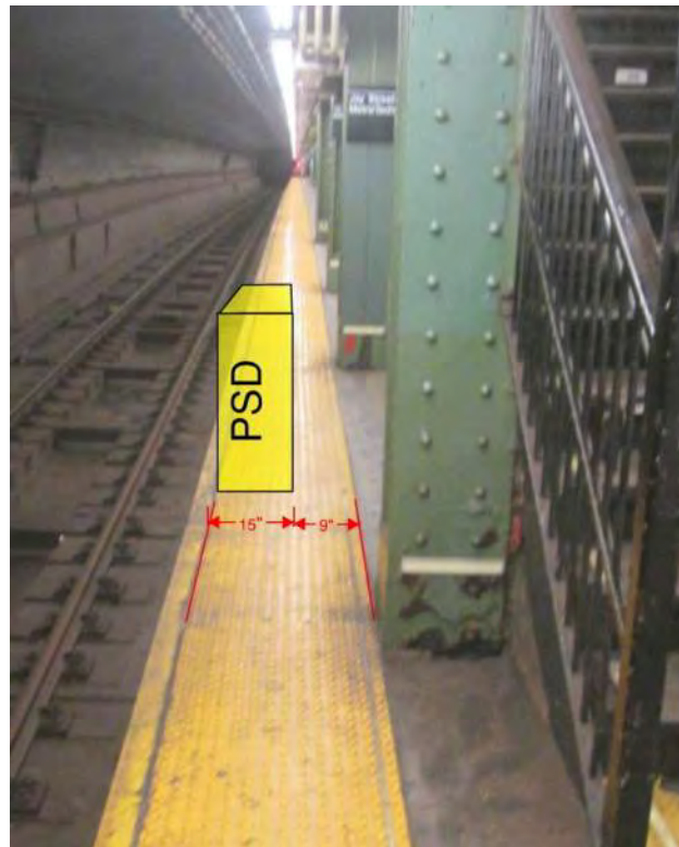
Figure 1 – Non-Compliant ADA condition Jay Street Station
