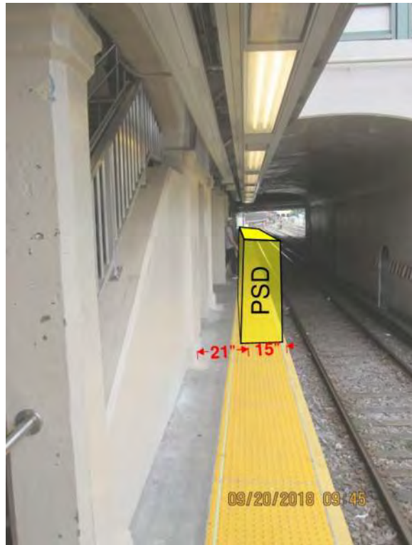
Figure 1 – Non-Compliant ADA condition 86 th Street Station
