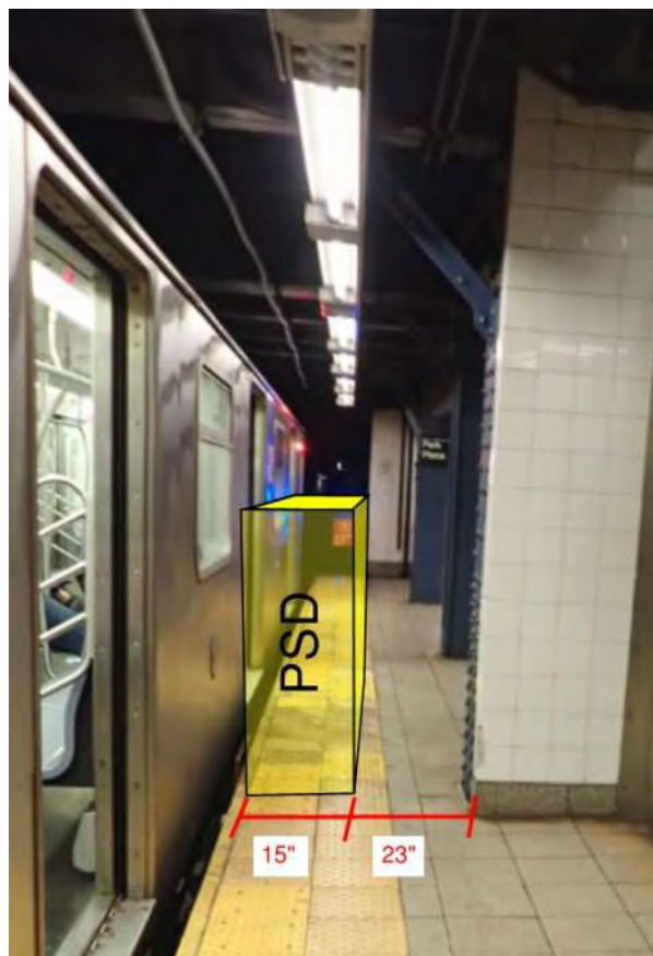
Figure 1 – Non-compliant ADA condition Park Place Station
