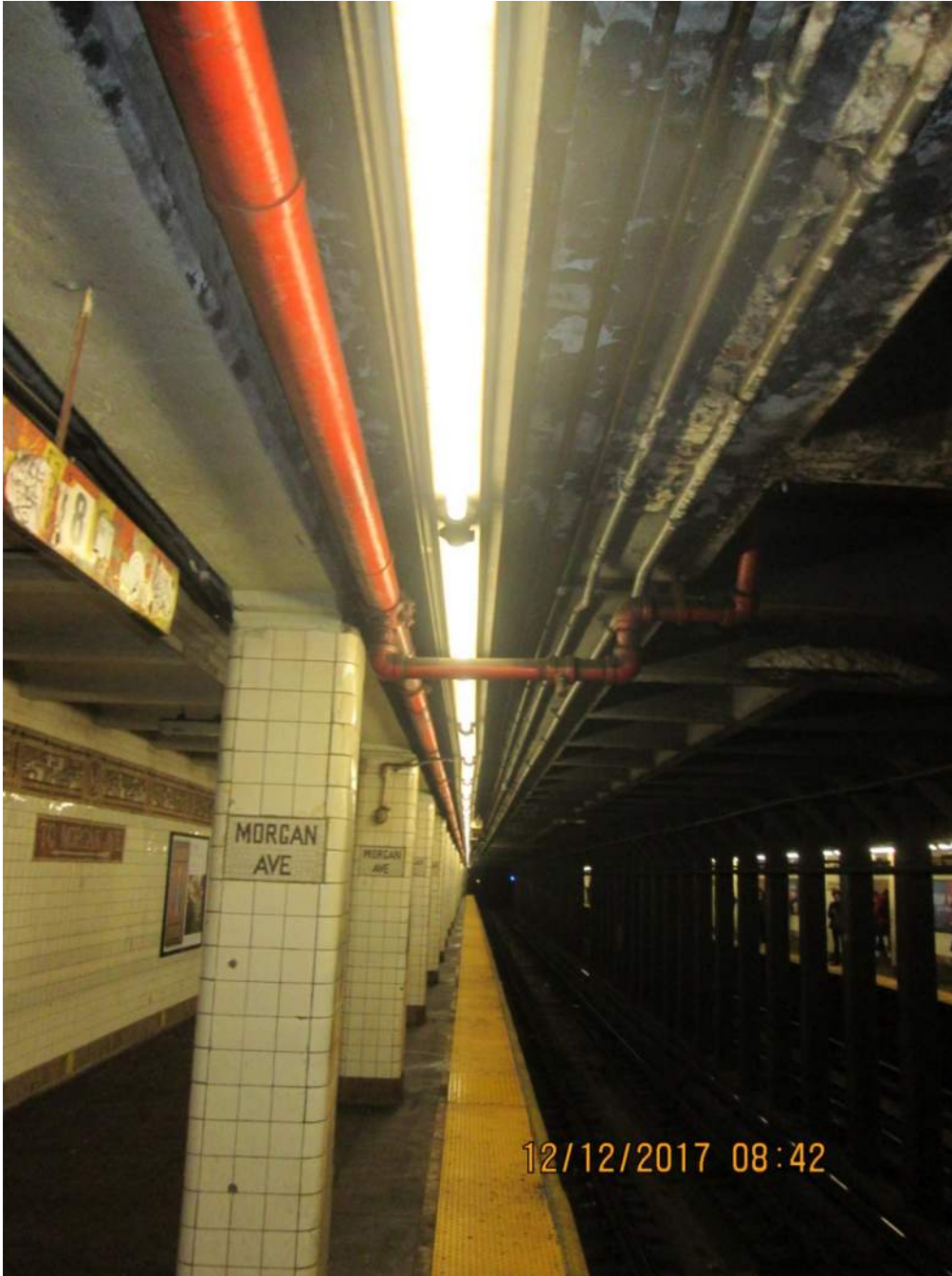
Figure 4 – Canarsie-bound Platform Standpipe Extending Beyond Platform Edge- Morgan Avenue Station
