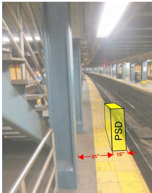
Figure 1 – Non-Compliant ADA condition Whitehall Street Station
