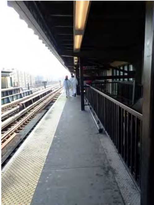
Figure 1 – General Station Condition Pelham Parkway Station
