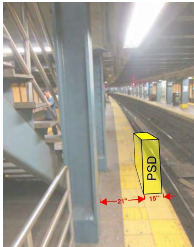
Figure 1 – Non-Compliant ADA condition Whitehall Street Station
