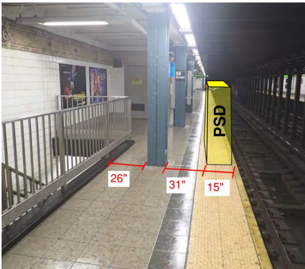
Figure 1 – Non-compliant ADA dimension 86 th Street Station- upper level
