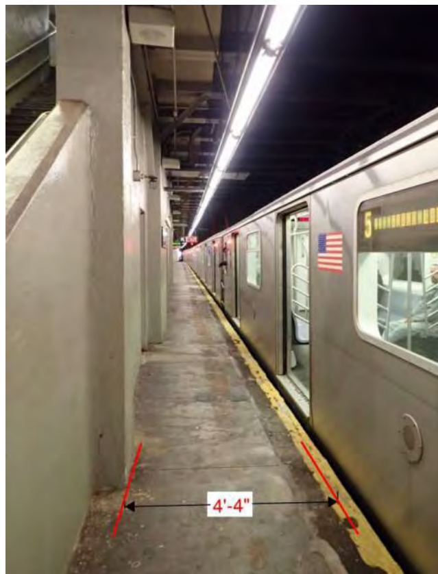
Figure 1 – Area of Non-compliant egress width Pelham Parkway Station
