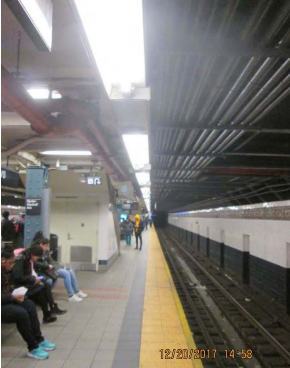
Figure 3 – Canarsie-bound: fire standpipe and conduit at/beyond platform edge– Myrtle Wyckoff Avenue Station
