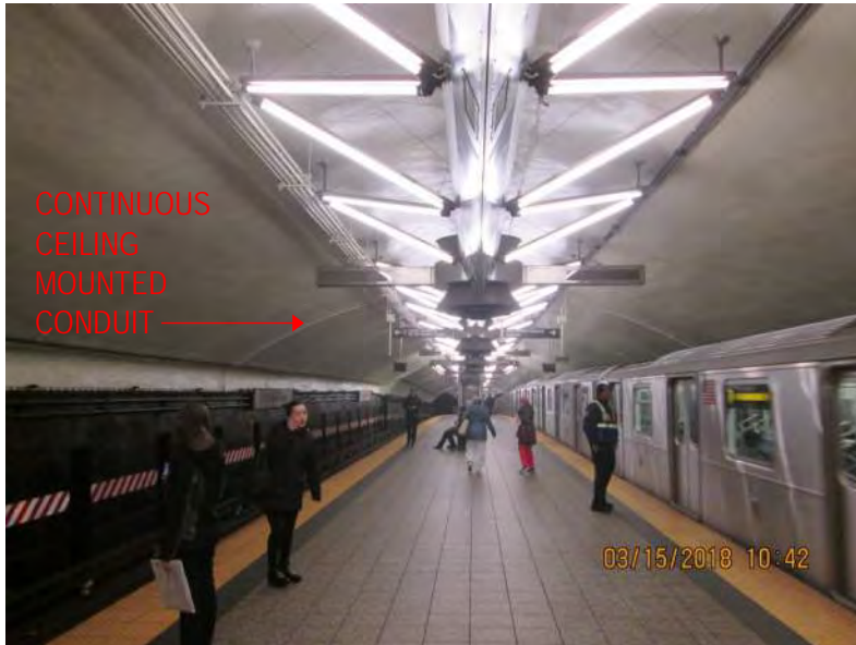
Figure 4– Typical platform view looking towards the end of the platform ends – 42 nd Street- Grand Central Station
