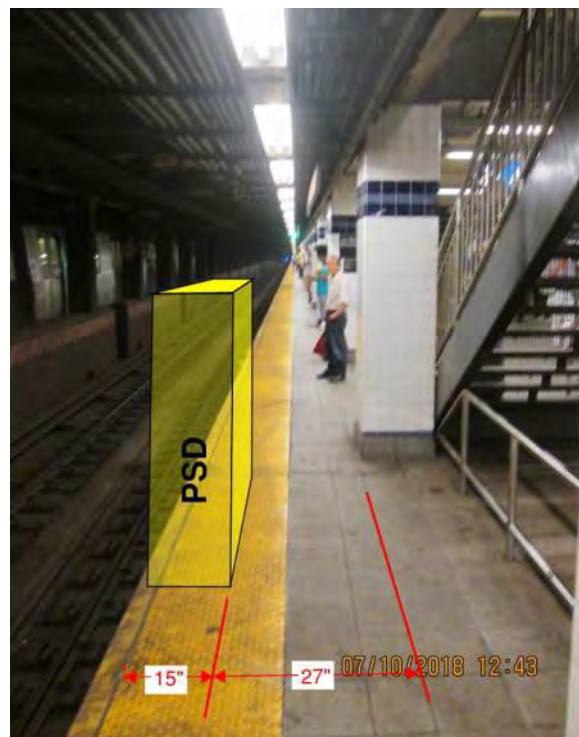
Figure 1 Non-Compliant ADA condition at stairs
