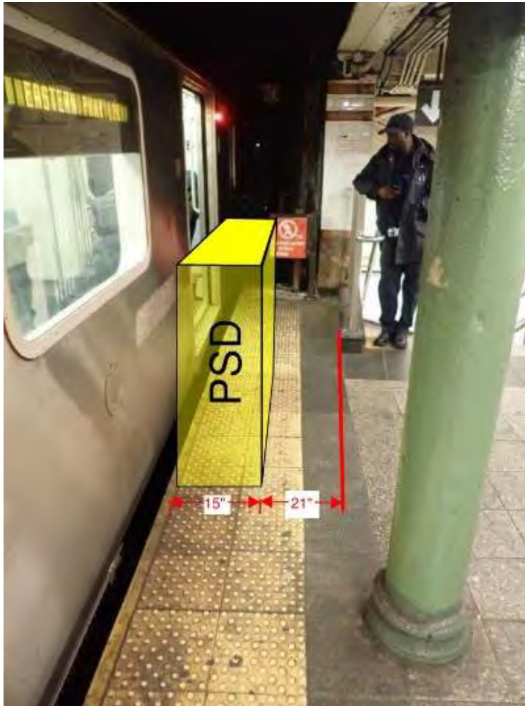
Figure 1 – Non-compliant ADA condition Atlantic Ave Station
