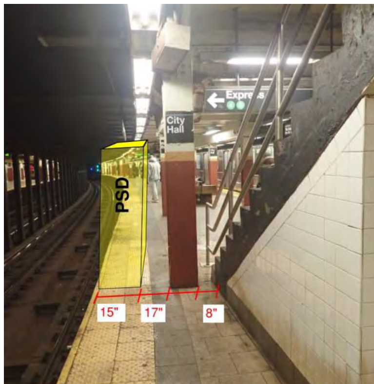
Figure 1 – Non-compliant ADA condition Brooklyn Bridge City Hall Station
