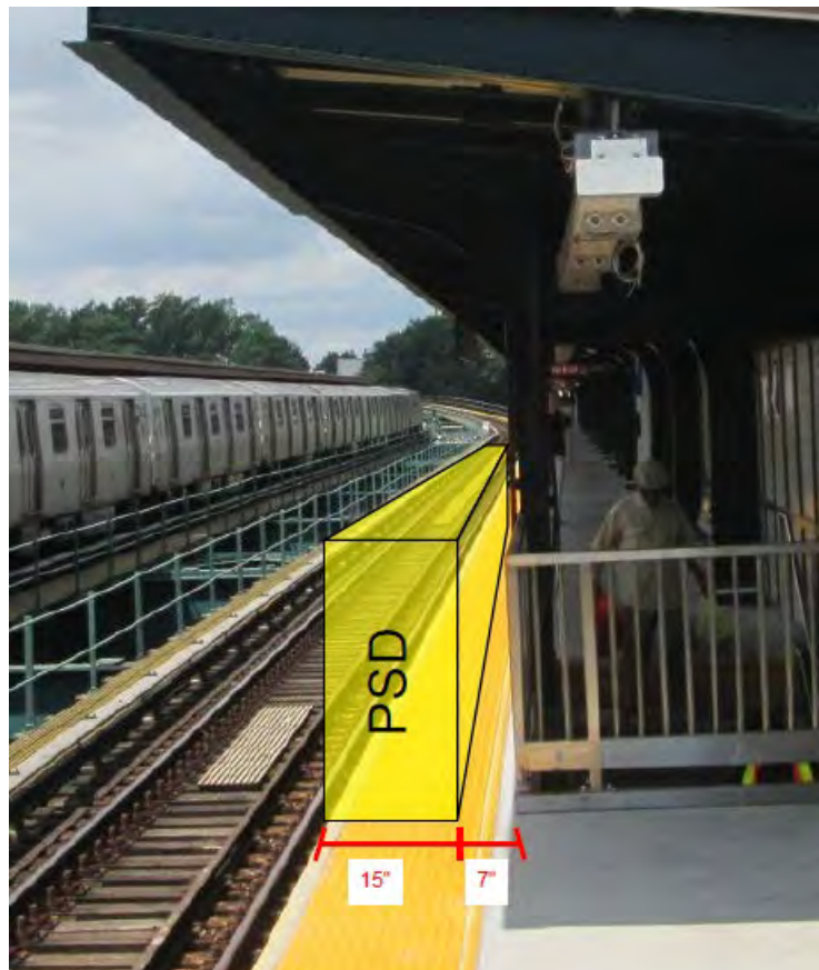
Figure 1 – Non-Compliant ADA condition 104 th Street Station
