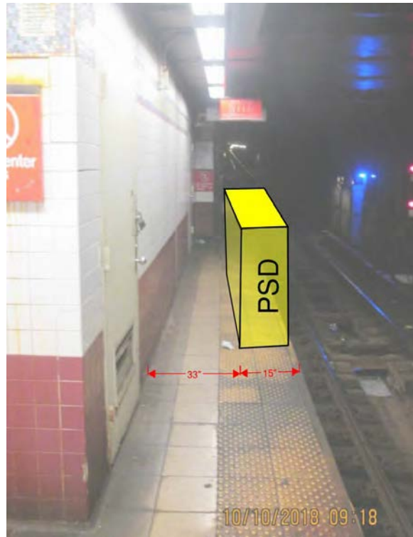
Figure 1 – Non-Compliant ADA condition Canal Street Station
