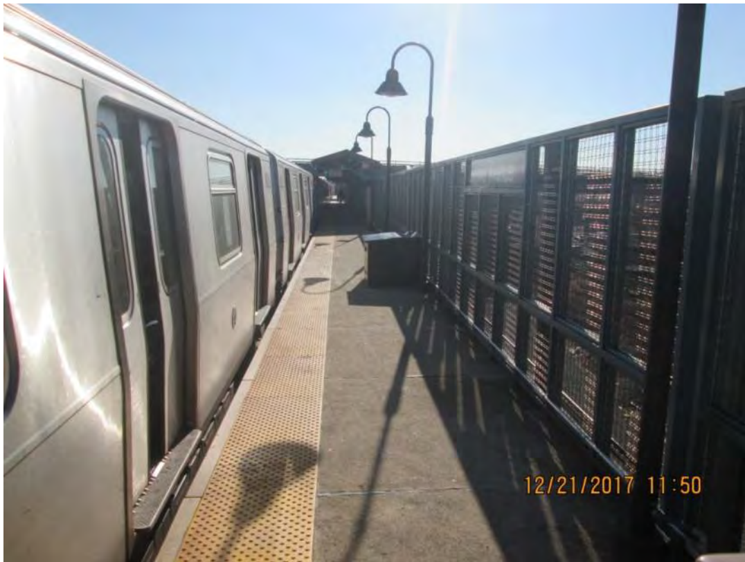
Figure 1 – Canarsie-bound platform, typical platform condition– Livonia Avenue Station
