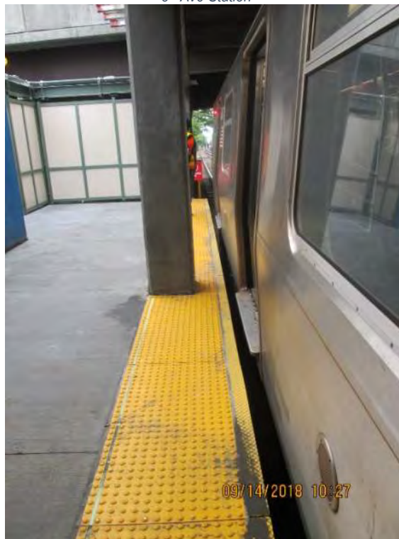
Figure 4 – Platform column (1 of 2) which will require removal and replacement 8 th Ave Station
