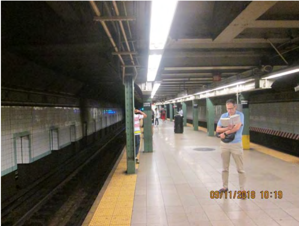
Figure 3 – View of column at platform edge requiring removal and replacement Atlantic Ave Station
