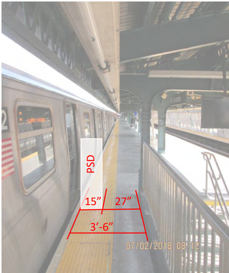
Figure 1– Non-compliant ADA condition – 18 th Avenue Station
