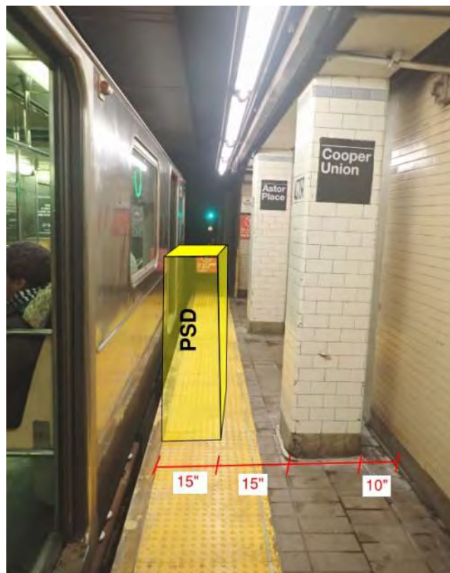
Figure 1 – Non-compliant ADA condition Astor Place Station
