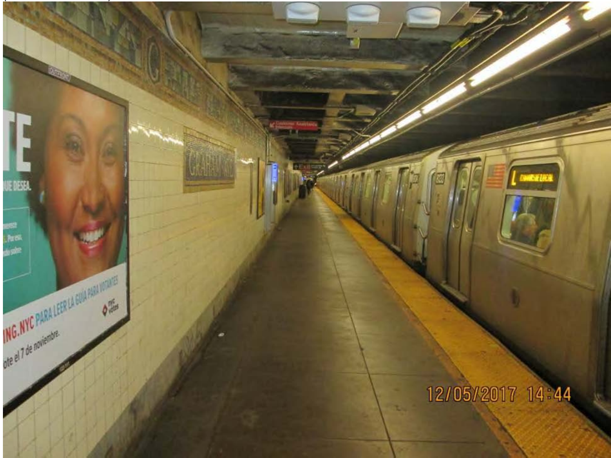
Figure 3 –Typical Platform Condition- Graham Avenue Station
