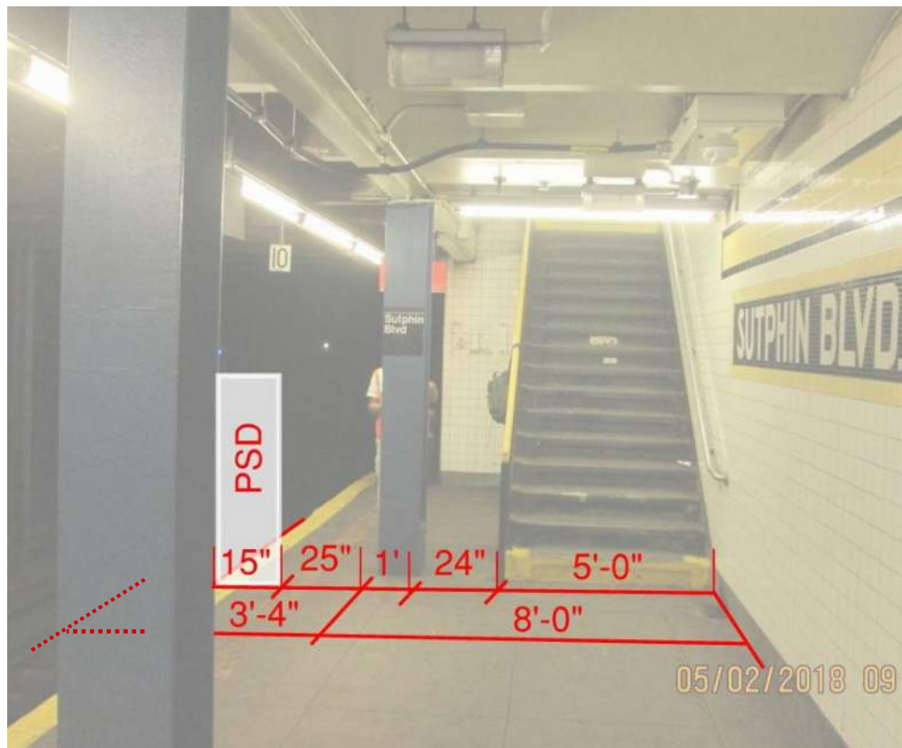
Figure 1 – Non-compliant ADA condition at stairs (typical)- Sutphin Blvd. Station
