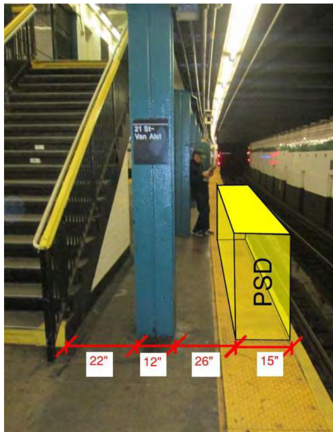
Figure 1 – Non-Compliant ADA condition at the platform edge adjacent to southernmost staircase on the southbound platform MRN 285: Metropolitan Avenue
