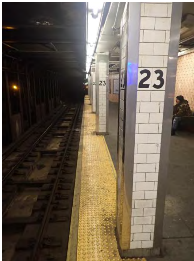
Figure 1 – Column 14” from the edge 23 rd Street Station
