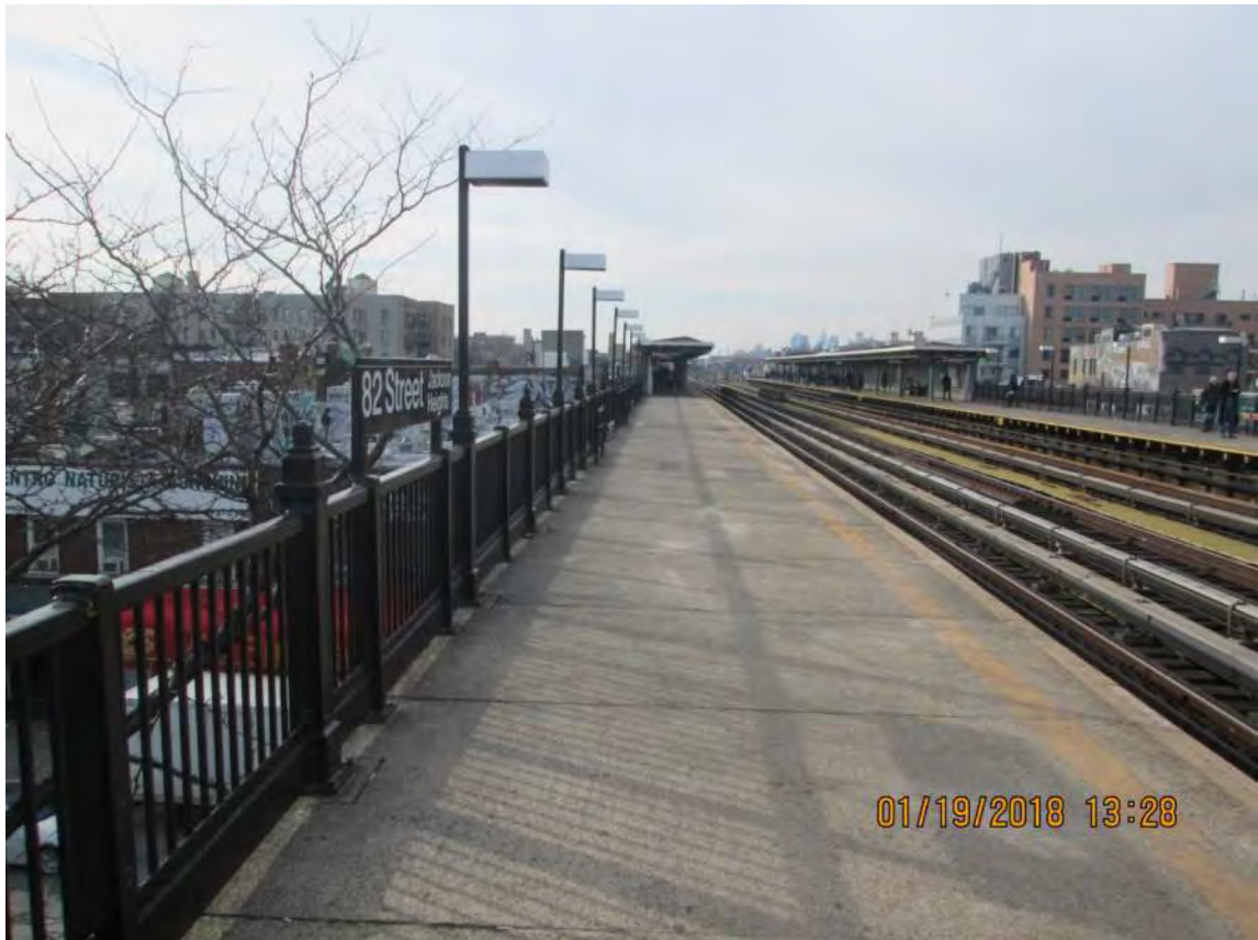
Figure 1 – Considerable Portion of the Platform Not Covered – 82nd Street-Jackson Heights Station
