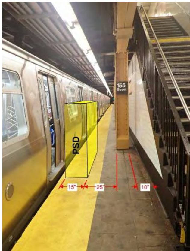
Figure 1 – Non-Compliant ADA condition 155 th Street Station
