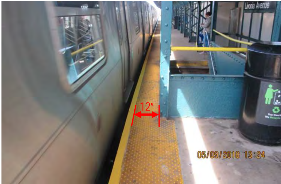
Figure 2 – Manhattan-Bound track platform, Staircase P3 is 12" away from platform edge – Livonia Avenue Station
