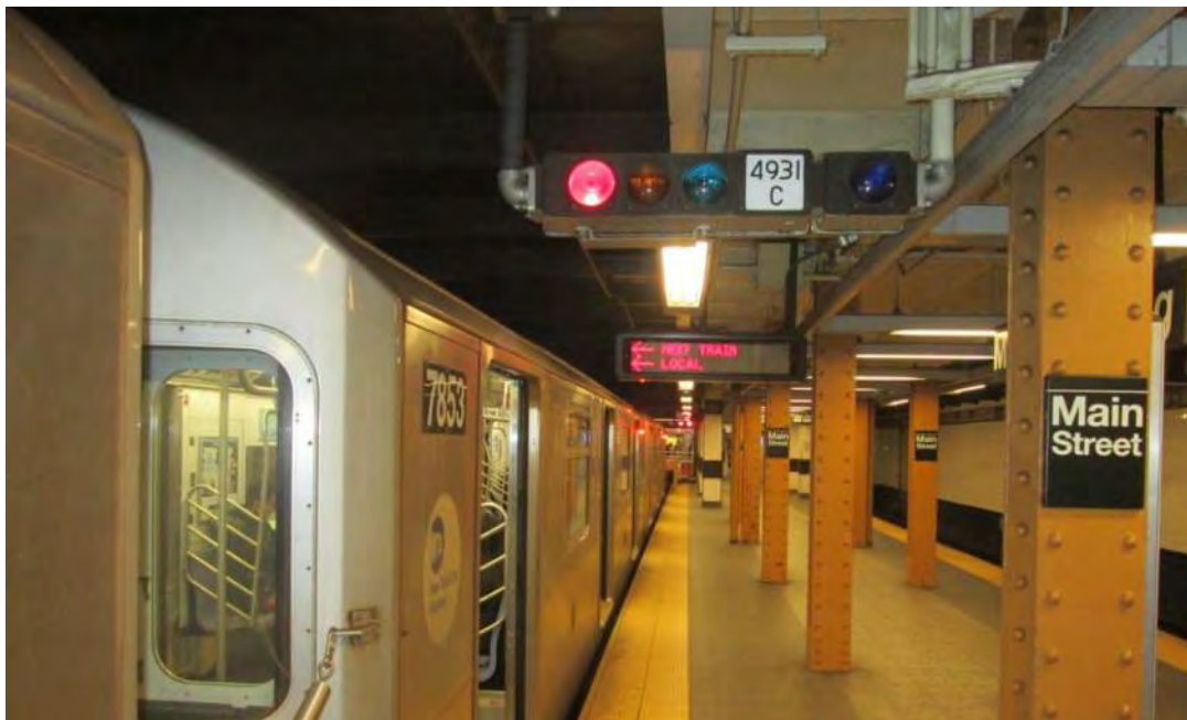
Figure 4 – Signal box at platform edge with a vertical clearance of 7'-6" - Flushing-Main Street Station
