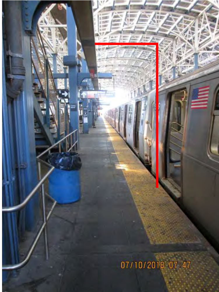
Figure 3 – Typical platform edge condition with line of potential supplementary framing Coney Island-Stillwell Avenue Station
