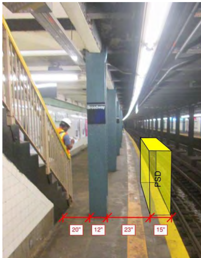
Figure 1 – Non-Compliant ADA condition at the platform edge adjacent to the underpass stairs MRN 288: Myrtle Willoughby Streets Station
