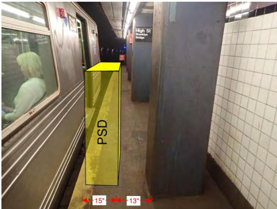
Figure 1 – Non-Compliant ADA condition High Street Station
