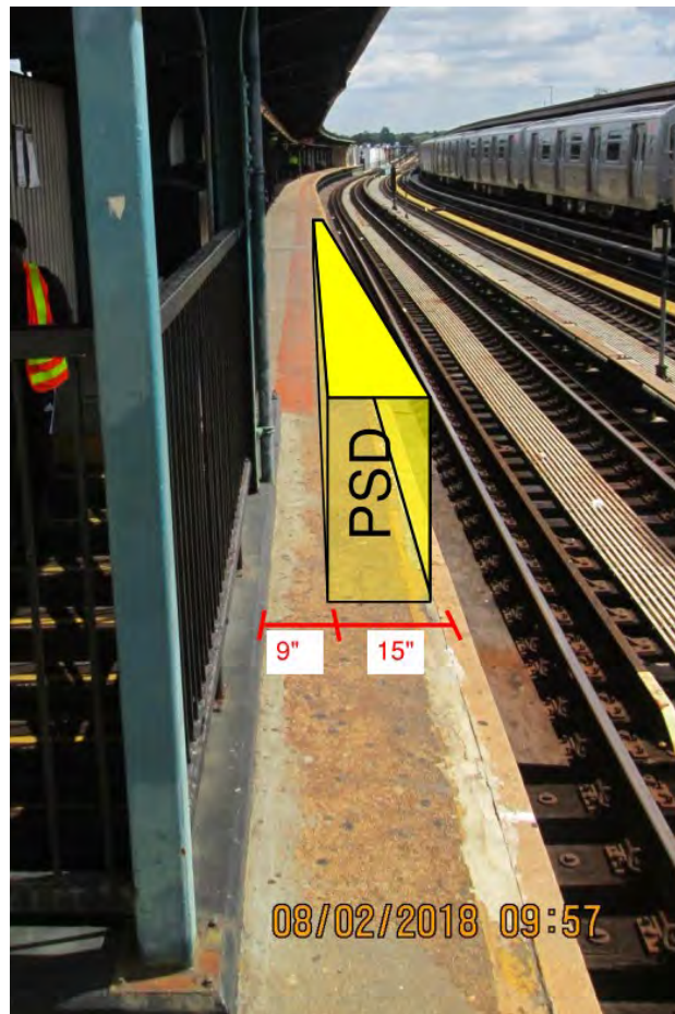
Figure 1 – Non-Compliant ADA condition 111 st Street Station
