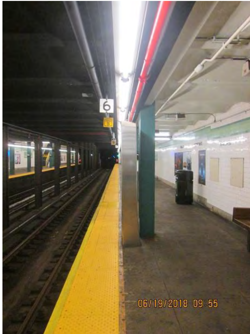
Figure 3 – Typical platform view with standpipe & free-standing monitor MRN 291 – Clinton & Washington Avenues
