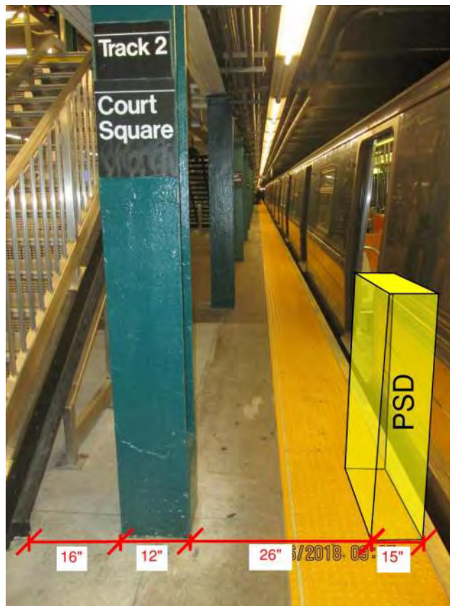
Figure 1 – Non-Compliant ADA condition MRN 281: Court Square
