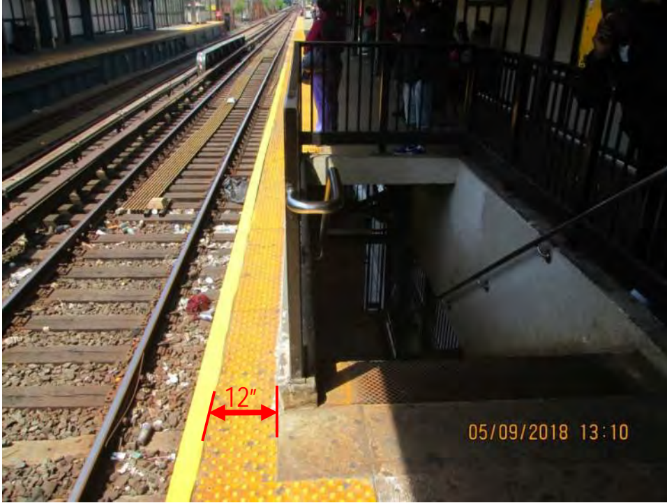
Figure 2– Manhattan-Bound track platform, Staircase P3 is 12" away from platform edge – New Lots Avenue Station
