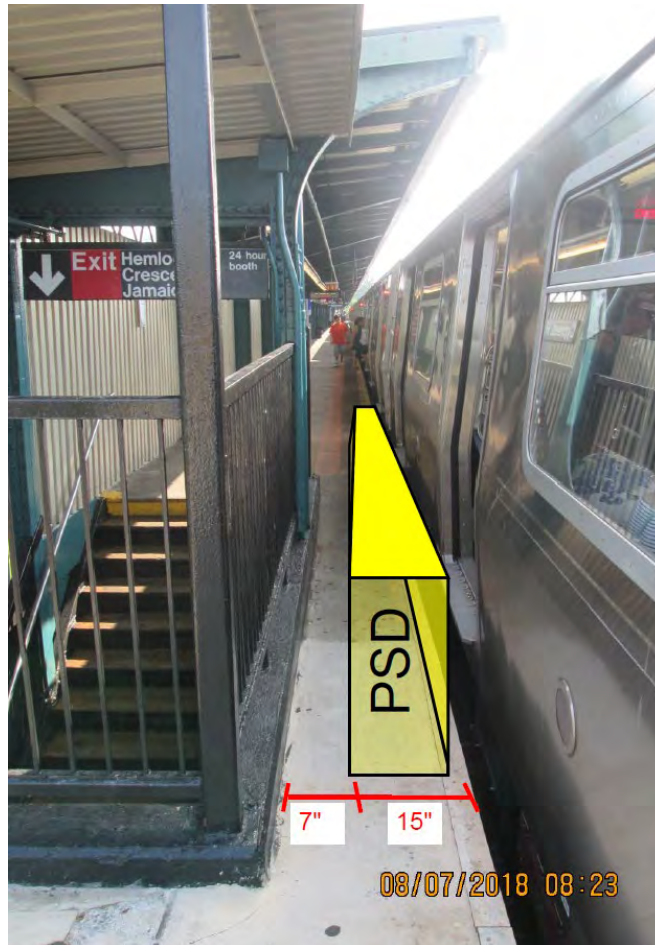
Figure 1 – Non-Compliant ADA condition Cypress Hills Station
