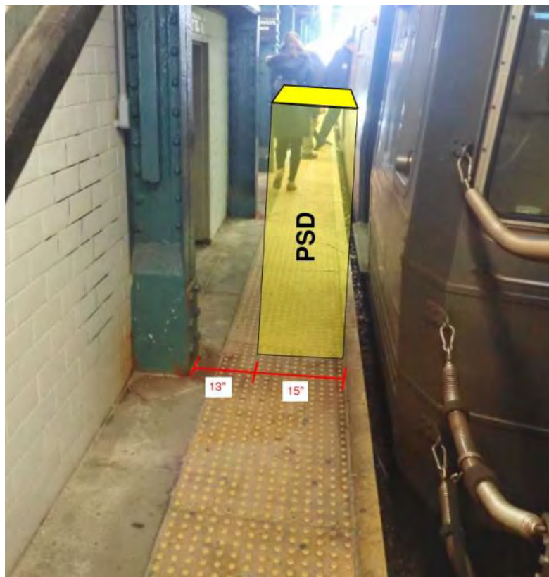
Figure 1 – Area of ADA non-compliance Newkirk Plaza Station
