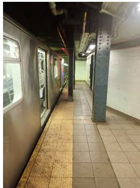
Figure 2 – Columns at 16” from platform edge South end of upper platform
