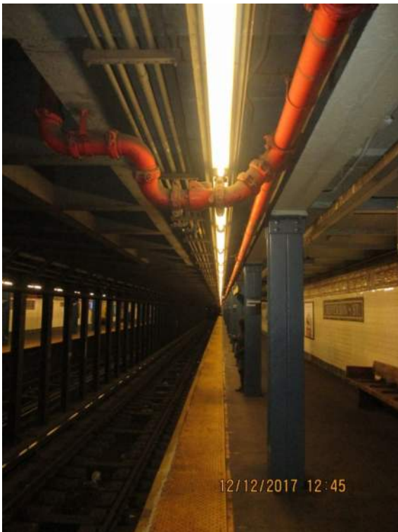
Figure 4 – Fire standpipe extending over platform edge with 7'-1" clearance (Manhattan-bound)—Jefferson St Station
