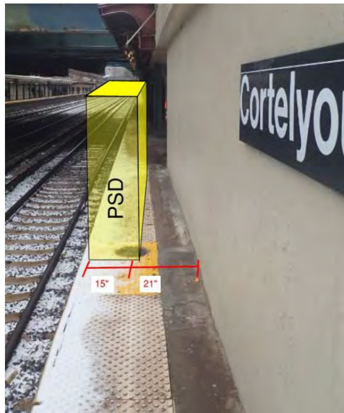
Figure 1 – Area of ADA non-compliance Cortelyou Road Station
