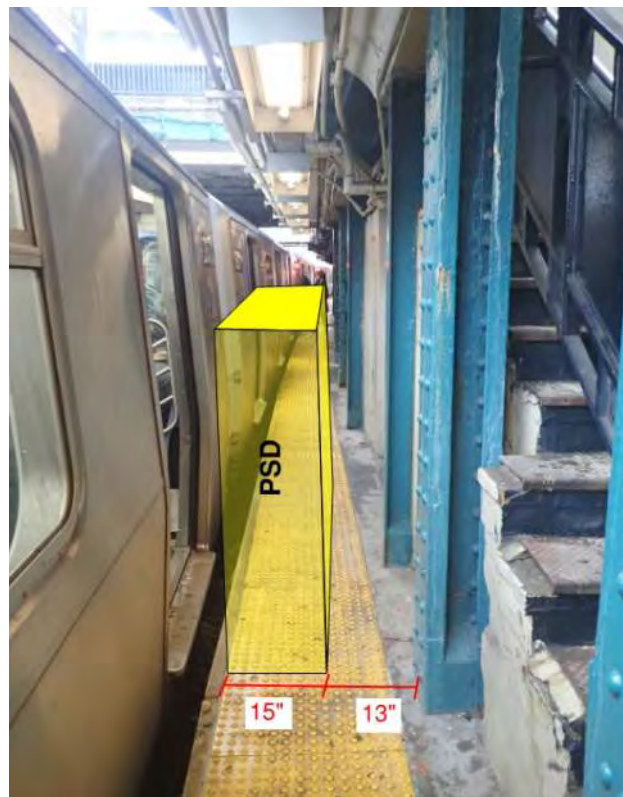
Figure 1 – Area of ADA non-compliance Beverly Road Station
