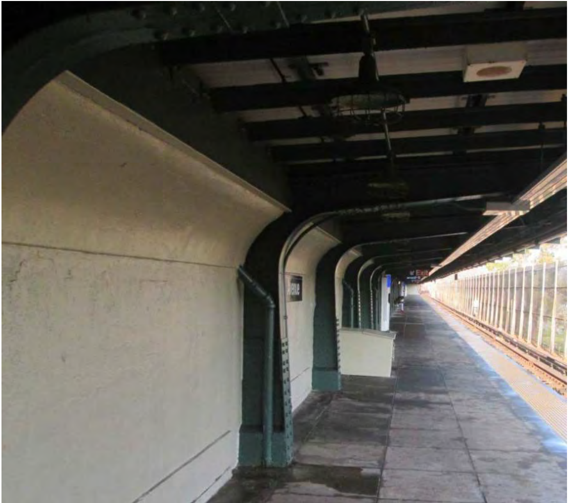
Figure 4 – Edge of Platform Condition, Canarsie-bound – Wilson Avenue Station
