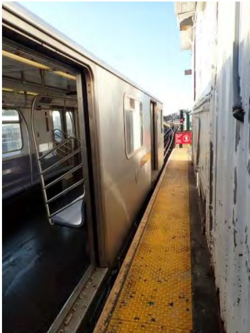
Figure 1 – Non-compliant ADA Condition 241 st Street Station
