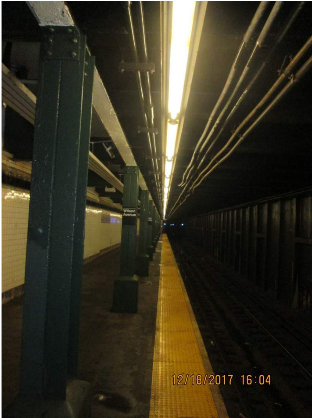
Figure 5 – Edge of Platform Condition, Manhattan-bound – Wilson Avenue Station
