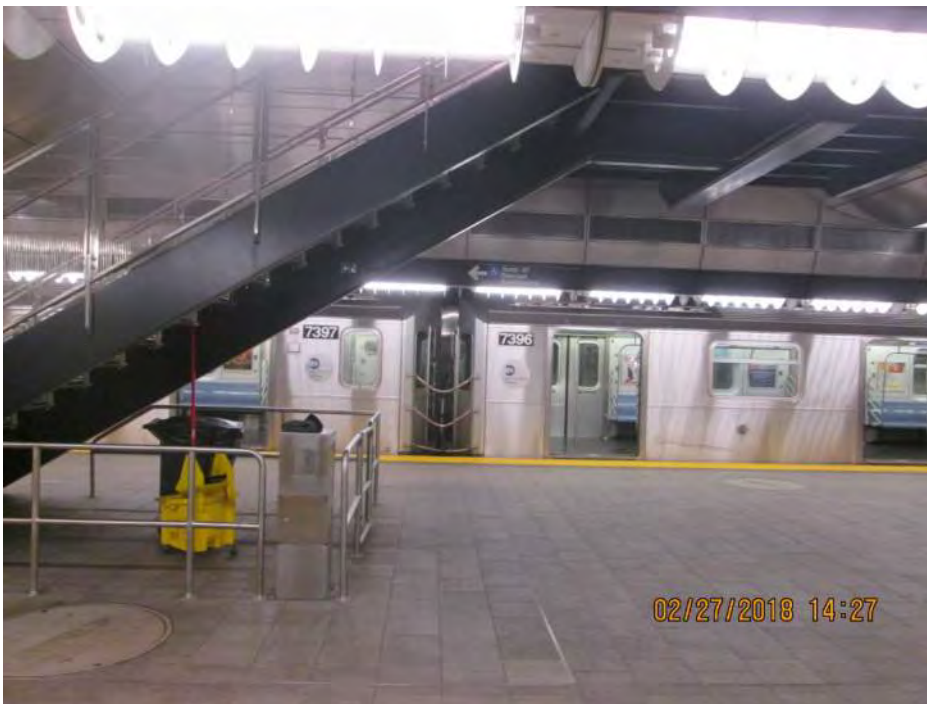
Figure 3 –Typical condition beneath stairs-34th Street- Hudson Yards Station
